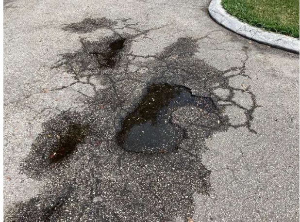
Pavement pothole formation
