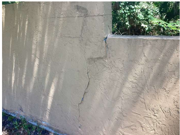
Wall stucco cracks
