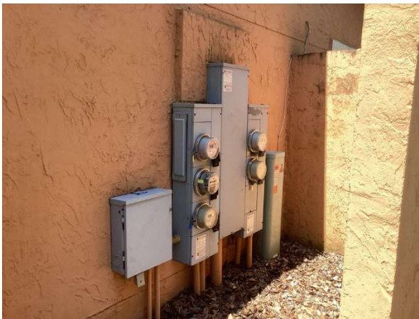
Electrical system main panels
