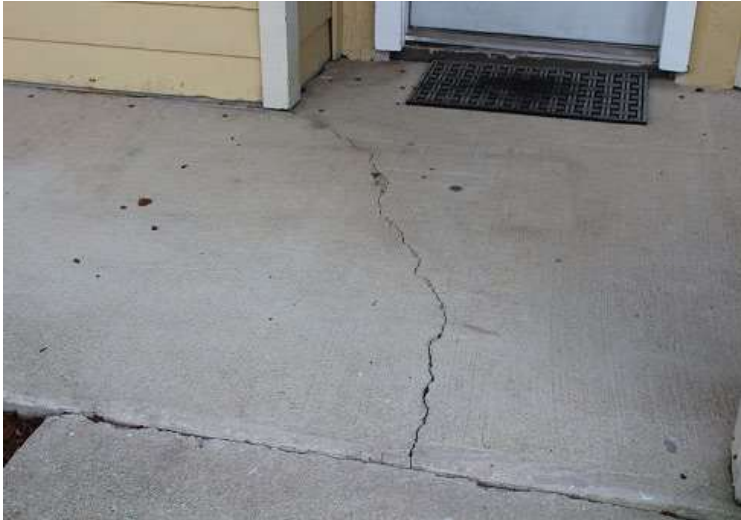
Typical sidewalk cracks near stairs
