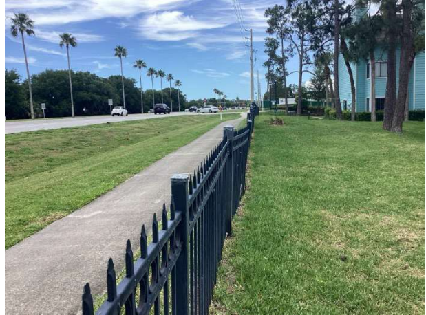
Fence leaning section
