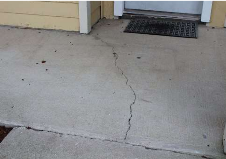
Typical sidewalk cracks near stairs
