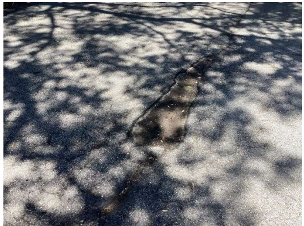
Pavement pothole formation
