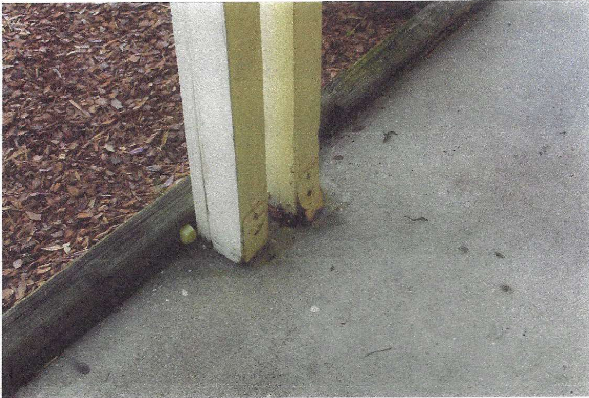
Posts on Front and Rear Porches Rotten Bases
