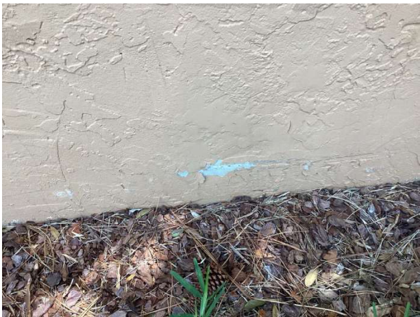
Wall paint finish deterioration
