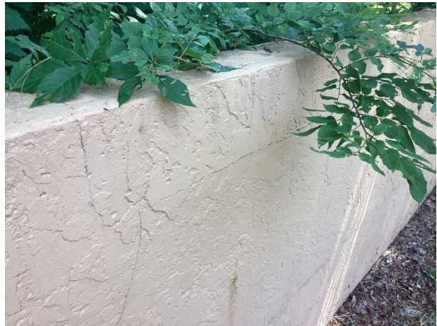
Wall stucco cracks
