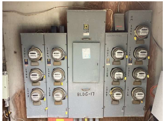
Electrical system main panels
