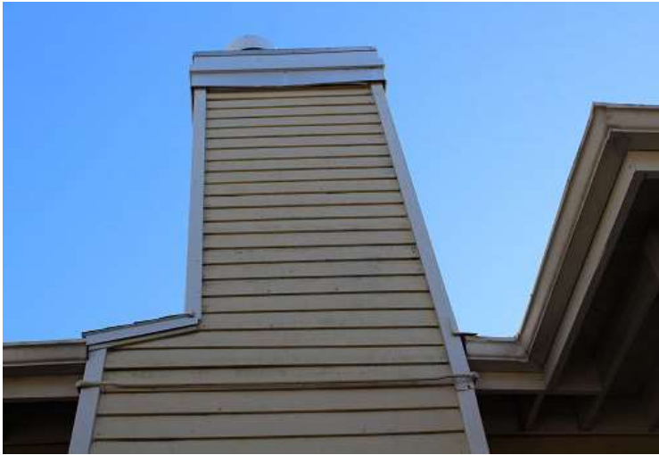
Chimney chase leaning
