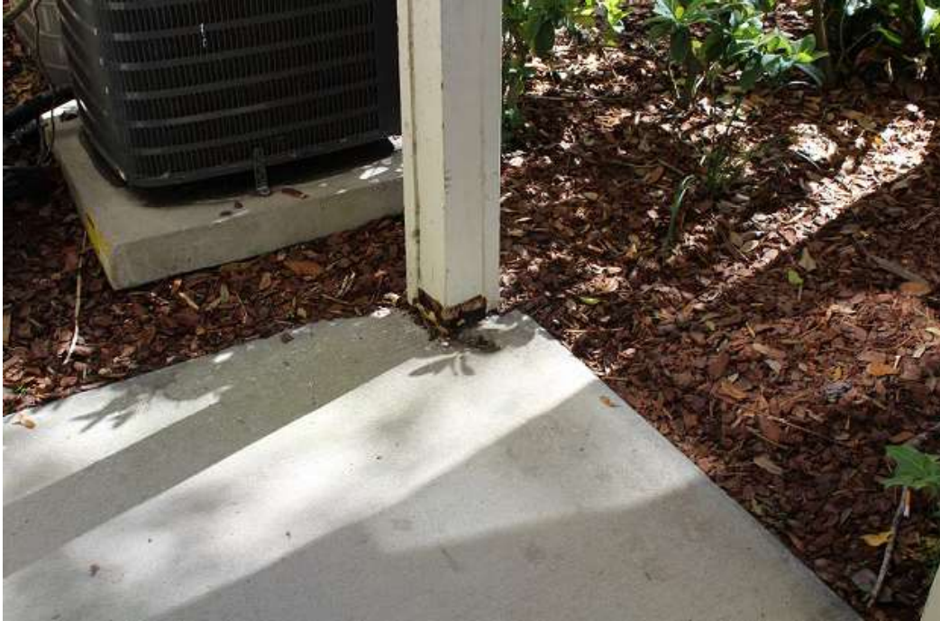
Rotten post base several locations
