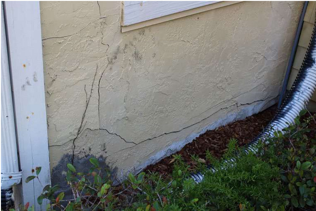
Stucco cracks next to west front chimney chase
